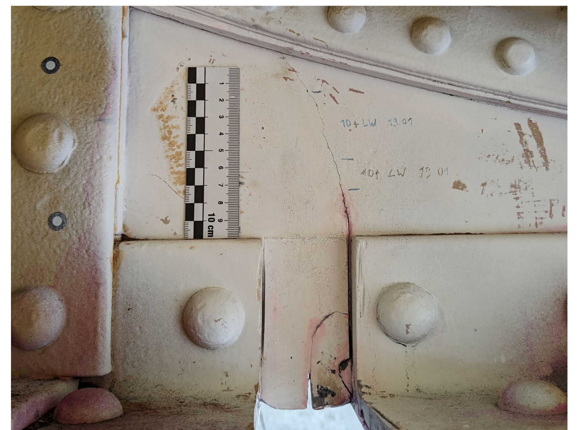
Fatigue crack caused by artificially induced damage
